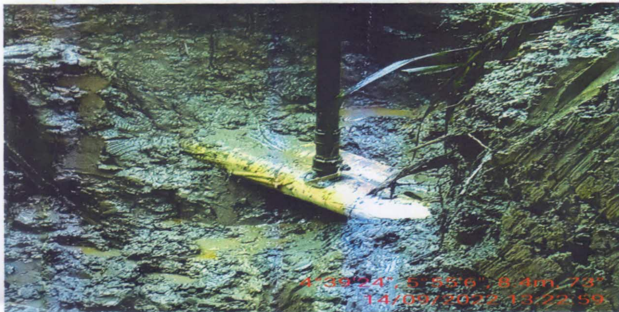
PICTURE 1: SHOWING 2" VALVE INSTALLED AT 12 O' CLOCK POSITION BY UNKNOWN PERSON FOR CRUDE OIL THEFT.
